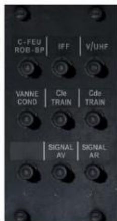
Figure 3Circuit breaker panel
